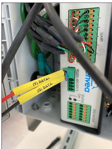
Figure 3-2 – RS485 cabling on IQ-LINK side
