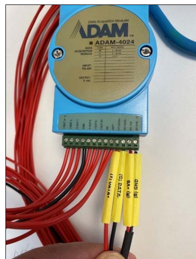
Figure 3-3 – RS485 cabling on ADAM side
